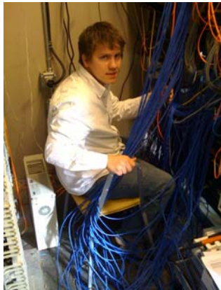
Jonathan Cox, a Subcontractor, Bundles Data Cables in Hut 1 During ITRP-2 Upgrades
