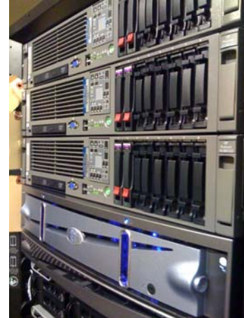
Virtual Servers and Storage Rack-mounted in Data Center
