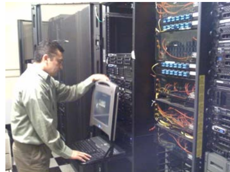
Walter Abarca at Console in Data Center's Equipment Room
